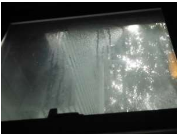
Figure 7 example of vapor seal breaks; have window installer Evaluate/repair and rule out any concealed damage by carpenter or building contractor.
