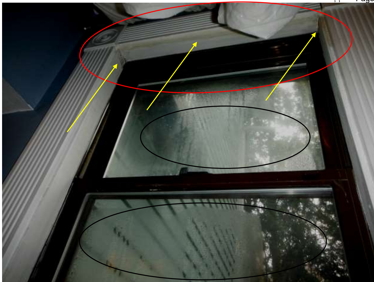
Figure 3 Water stains/leaking around window frame and vapor seal breaks; have window installer evaluate and carpenter evaluate window and advise on all damage & repairs. See window section comments.
