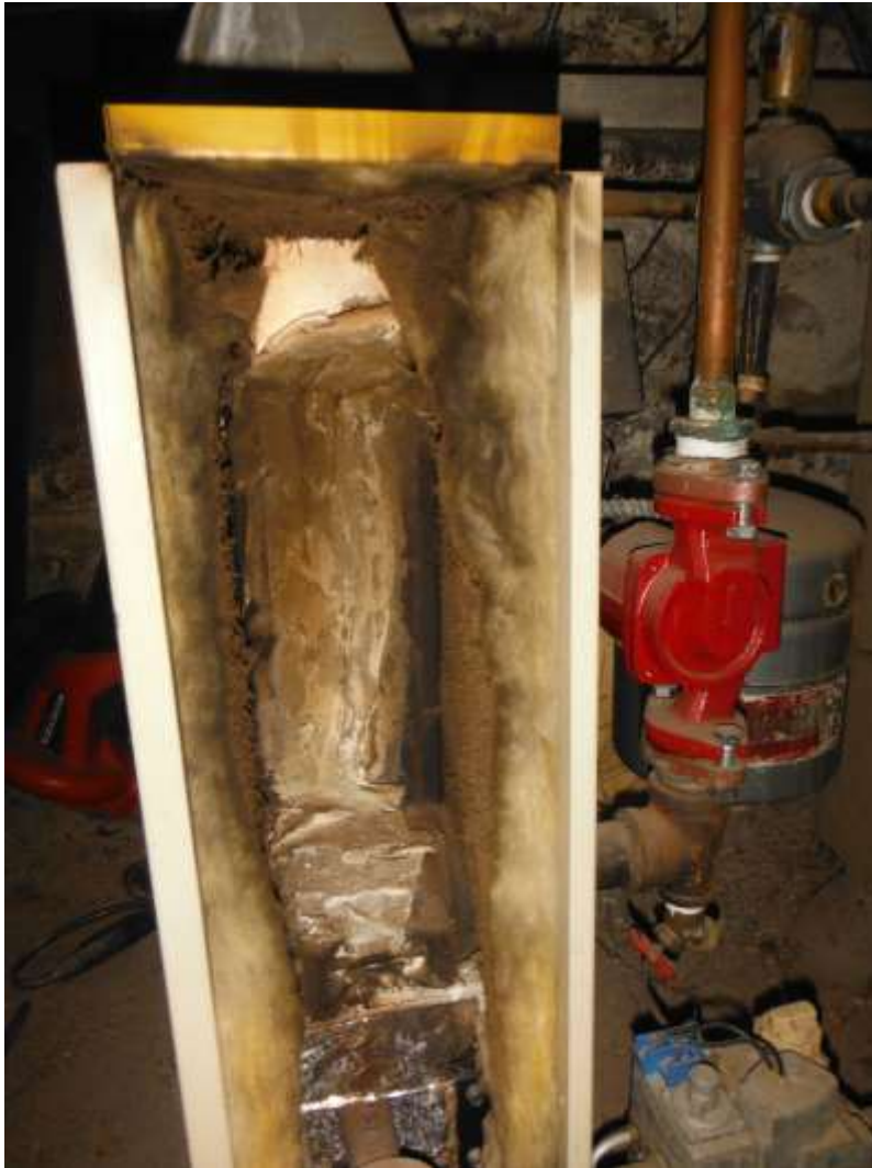
Figure 6 Poorly maintained boiler; have a boiler evaluate boiler and advise on repairs/replacement.
