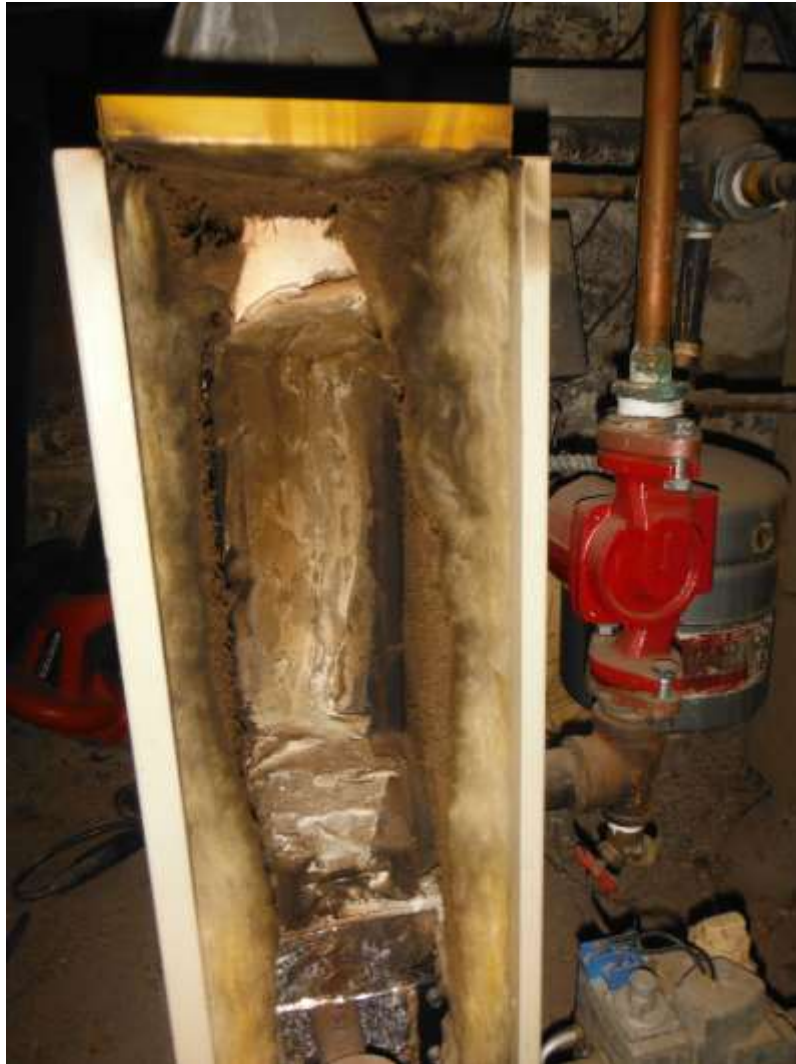
Figure 6 Poorly maintained boiler; have a boiler evaluate boiler and advise on repairs/replacement.
