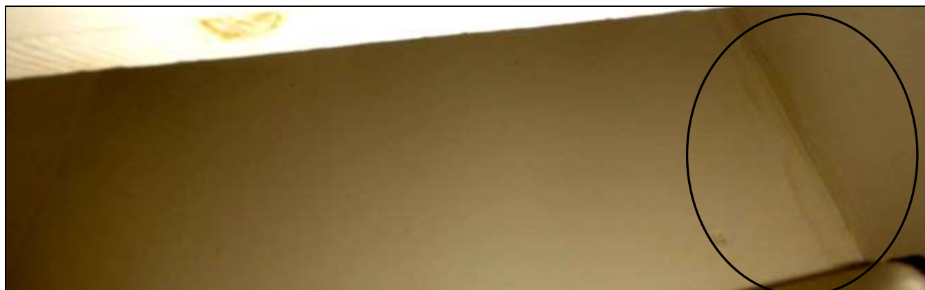
Figure 13 Water stains observed in interior of home especially around chimneys or adjacent to them. Have a roofer or building contractor evaluate all water sources and make repairs. Follow-up with Co-op to see who is responsible for exterior. Roof, gutters, flashings, etc. should be evaluated to determine all sources of leaking.
