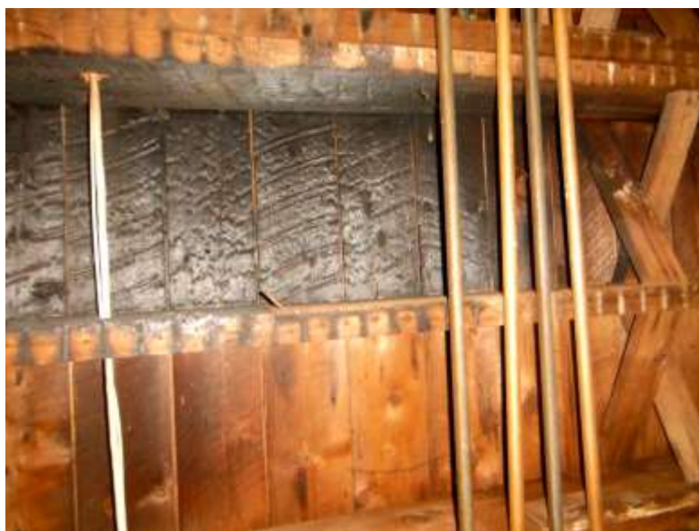
Figure 16 Observed fire damage in basement in common areas; follow up with the Association for fire damage.
