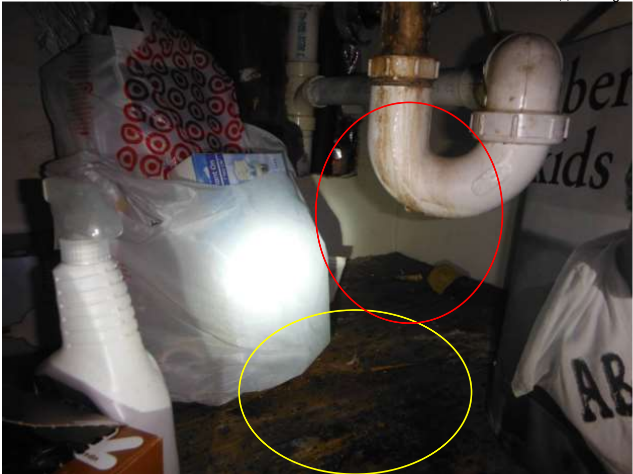
Figure 9 Leaking under sink from sink drain basket (heavily puttied), and drain assembly; have licensed plumber evaluate and repair. Have dark staining on cabinet bottom shelf further evaluated for mold. Identification, testing, and inspection of environmental or mold hazards is beyond the scope of a home inspection.
