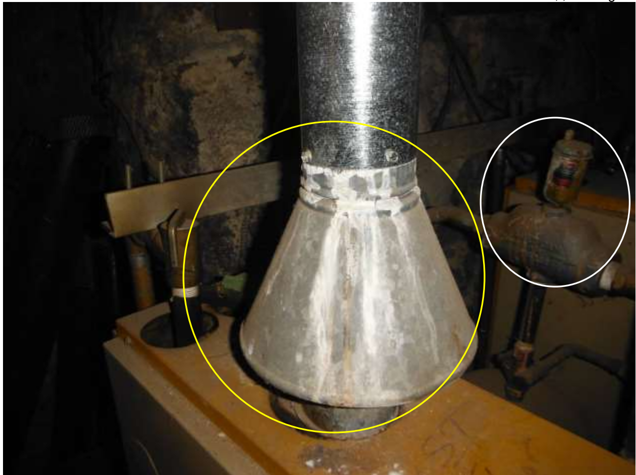
Figure 17 White condensate residue; drafting/safety concerns. Rust, leaking air vent, soot, etc.; poorly maintained boiler. Have a boiler contractor service and make repairs; boiler near or past expected life.
