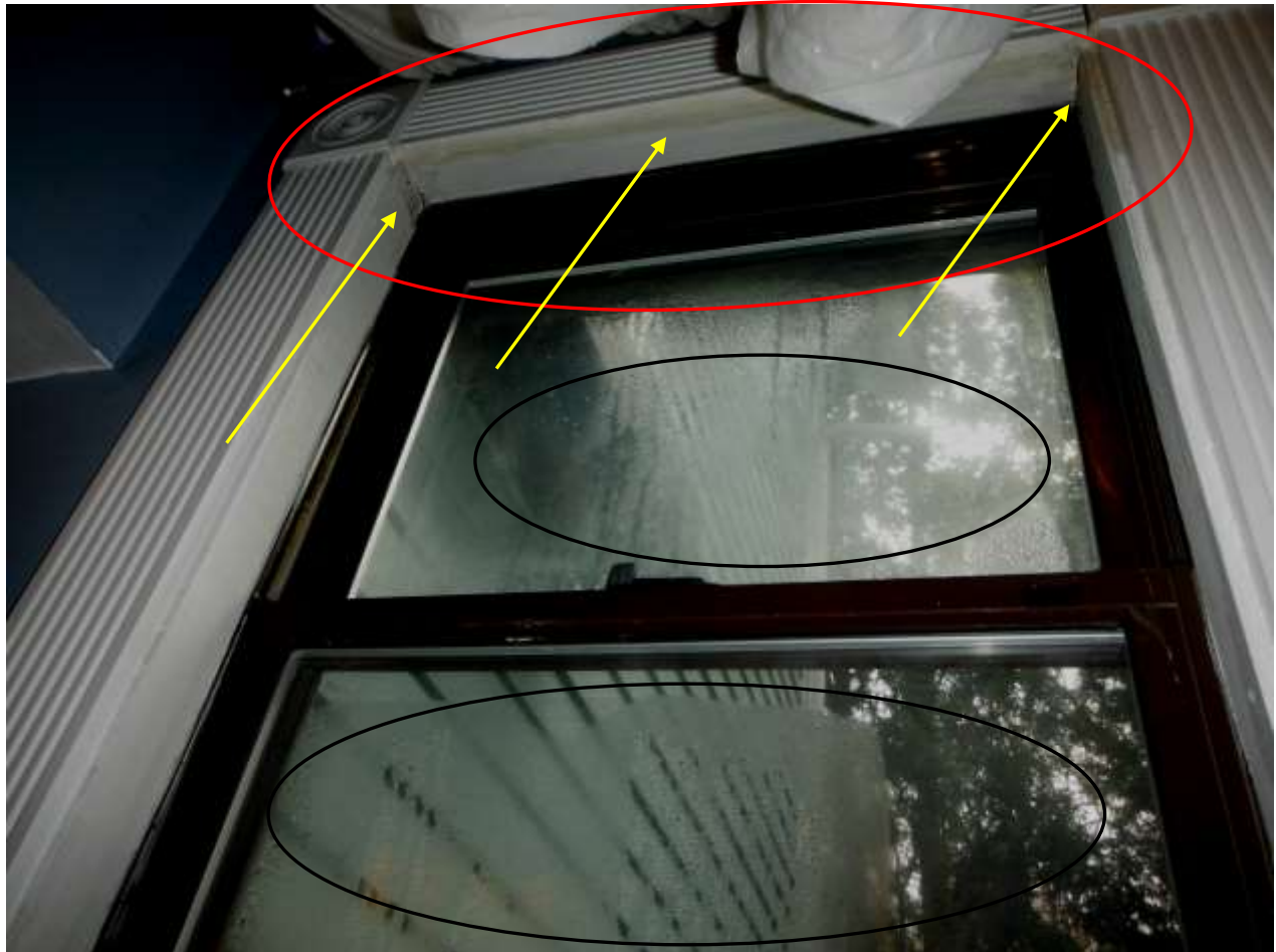
Figure 11 Water stains/leaking around window frame and vapor seal breaks; have window installer evaluate and carpenter evaluate window and advise on all damage & repairs. See window section comments.
