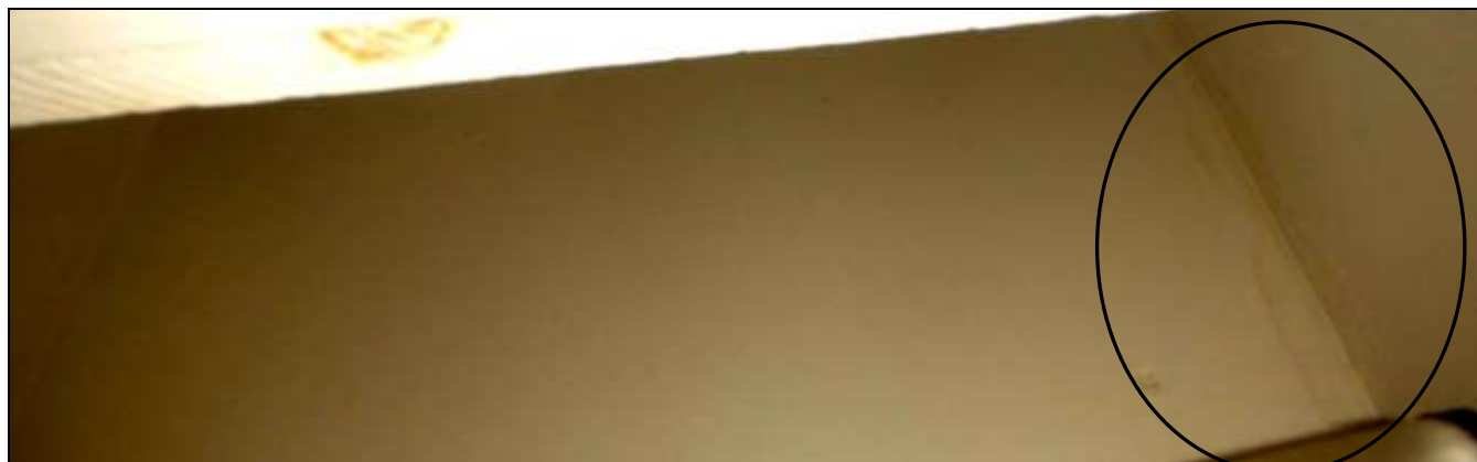
Figure 5 Water stains observed in interior of home especially around chimneys or adjacent to them. Have a roofer or building contractor evaluate all water sources and make repairs. Follow-up with Co-op to see who is responsible for exterior. Roof, gutters, flashings, etc. should be evaluated to determine all sources of leaking.
