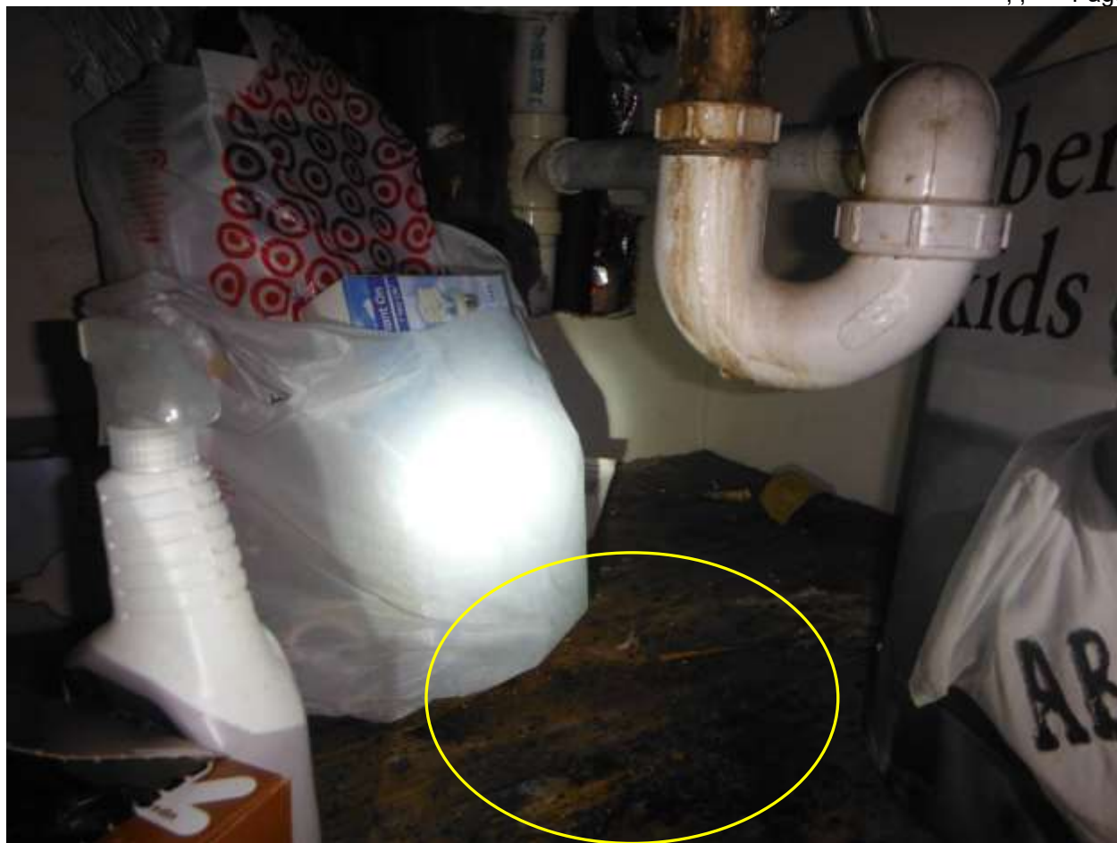
Figure 1 Leaking under sink from sink drain basket (heavily puttied), and drain assembly; have licensed plumber evaluate and repair. Have dark staining on cabinet bottom shelf further evaluated for mold. Identification, testing, and inspection of environmental or mold hazards is beyond the scope of a home inspection.
