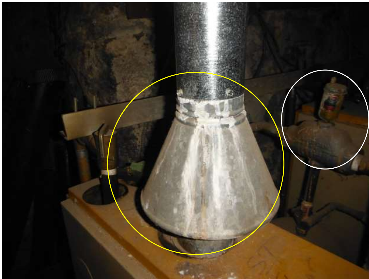
Figure 8 White condensate residue; drafting/safety concerns. Rust, leaking air vent, soot, etc.; poorly maintained boiler. Have a boiler contractor service and make repairs; boiler near or past expected life.
